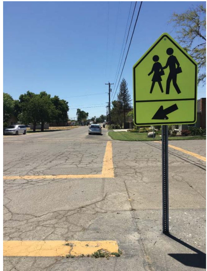
Crosswalk lacking adequate sidewalks and curbs in Riverdale.
